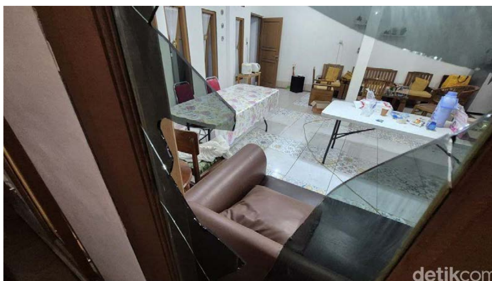
Figure 1. Physical Damage at Villa Ninna Following the Cidahu Religious Intolerance Incident
